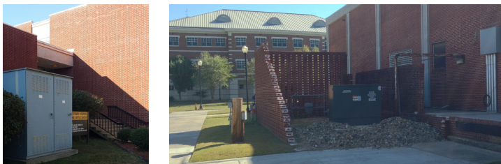
Figure 4.2-4, Examples of Existing Electrical Utilities around Campus
