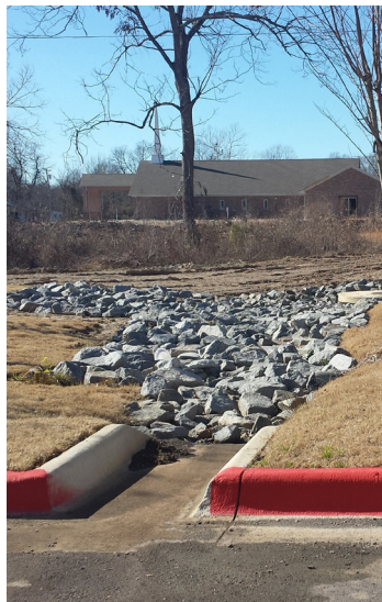
Figure 4.6-3, UAPB Stormwater Rip-Rap
